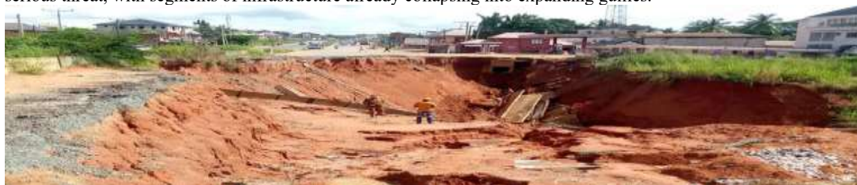
Figure III: An image showing the impact of gully erosion in Agulu-Nanka area in Anambra
