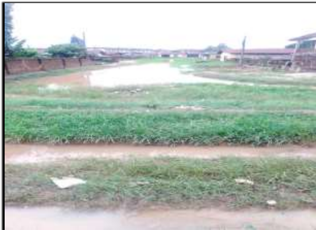
Plate 1: Clogged Earth Road with Flood Pondages and Plants Recovery at Edaiken Avenue by Uselu Traditional Grounds Source: Authors' Field Survey, 2023.
